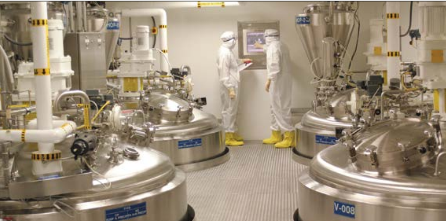
Focused on large-scale fractionation, Covington’s process galleries will look very similar to operations at its Los Angeles facility shown here.
