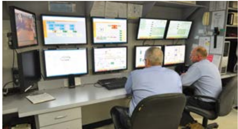
Figure 2. Virtualization can reduce the required number of PCs by 50% or more, while still providing all of the functionality of a traditional system, including multiple simultaneous views into various applications.
